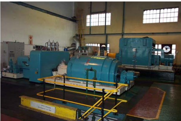
Pict. 20: Steam turbines / electricity generation
