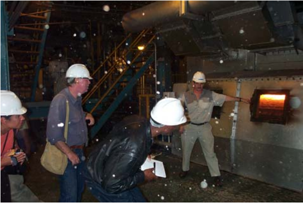
Pict. 18: Boiler for steam generation
