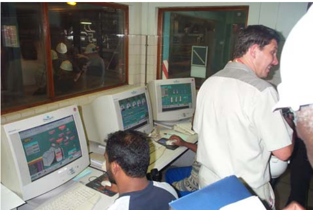
Pict. 19: Monitoring/control station of the boilers
