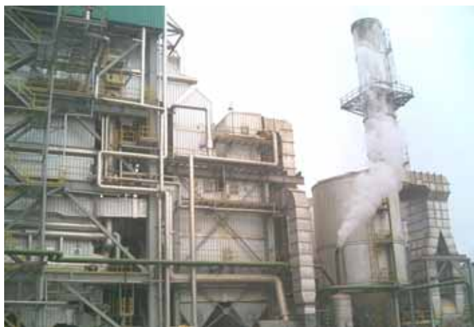
High pressure boilers at the Companhia Energética Santa Elisa
