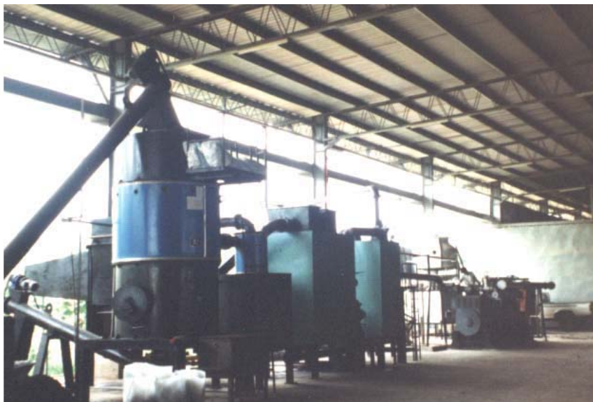
Fixed Bed Gasification - Electricity Generation Set Equipped with a Gas Engine
