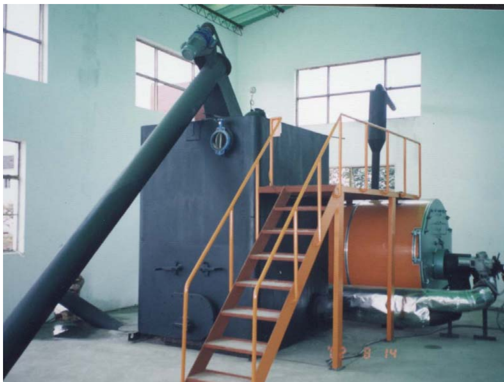
Photo of 1.4MW straw gasification-heating set
