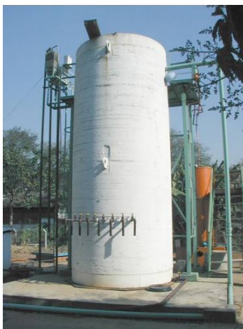
Figure 1 - Biodigestor Model UASB (Up flow Anaerobic Sludge Blanket)
