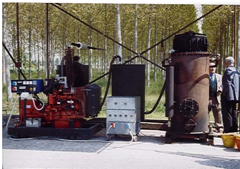
Fig. 1: Gasifier, gas filtration system and generator set
