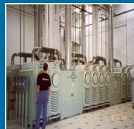
World's largest Microturbine Tri-generation project (540 kW), USA
