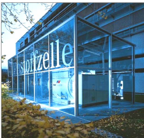
MTU HotModule installed at an office building in Munich
