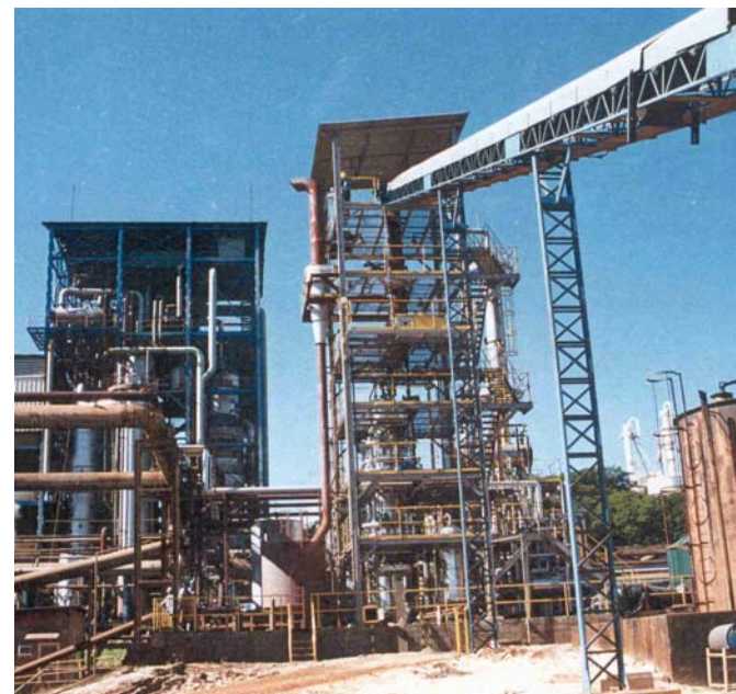
REACTOR TOWER WITH BAGASSE FEEDING SYSTEM
